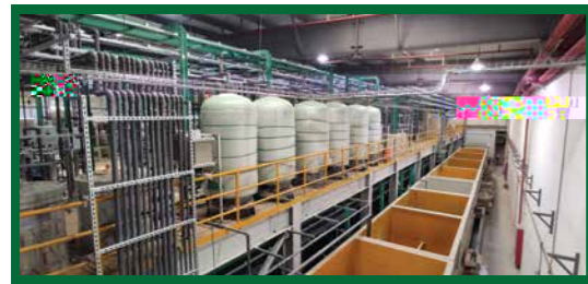
Domestic sewage Bar Screen / Grit Chamber Equalization Tank / Biochemical Tank / MBR Pump Clean Water Tank / Disinfection Reuse
